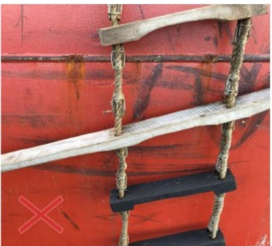
Loose ladder steps & not horizontal
