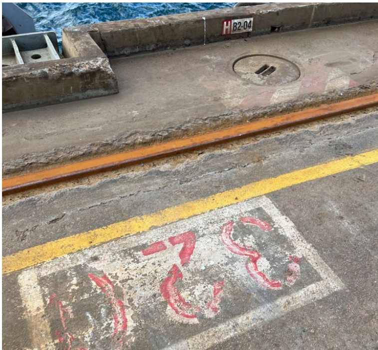
Figure - 7. Water hydrants between 310 to 360m mark on berth 2 are B2-04 and B2-05. Ensure the modified hatch over is used (refer to Figure 8).
