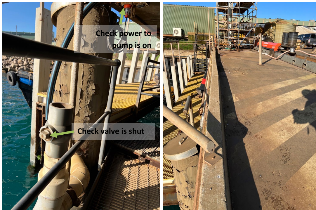
Figure 2 - Berth outlet valve shown in closed position to divert water to tanks
