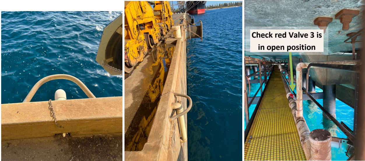
Figure 1 Berth scuppers and down pipe network under berth leading to sump
