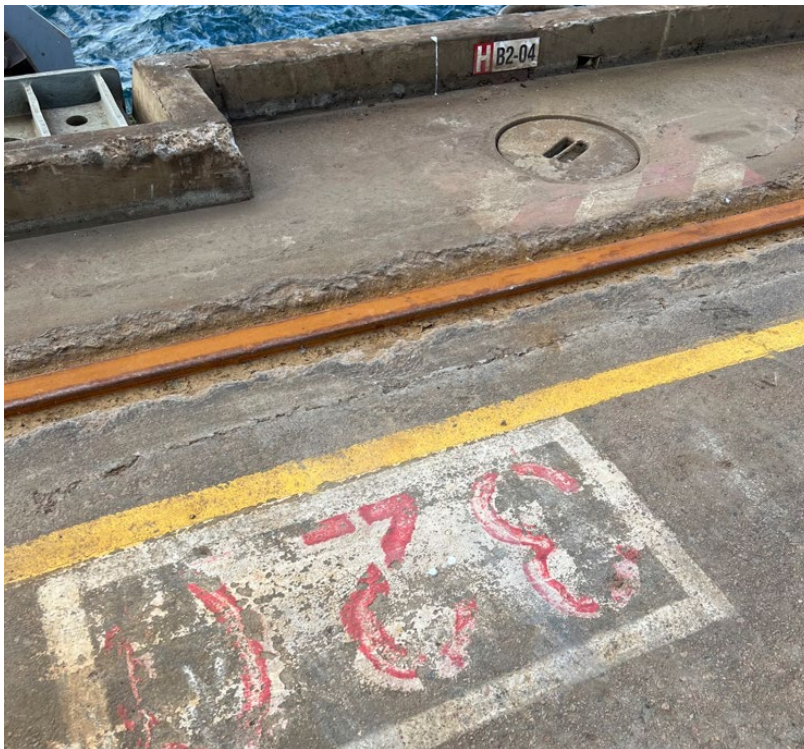
Figure 7. Water hydrants between 310 to 360m mark on berth 2 are B2-04 and B2-05. Ensure the modified hatch over is used (refer to Figure 8).
